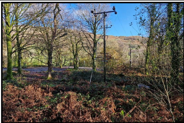
Photograph 11: Compartment 3. Overhead HV cable through southern part of group
