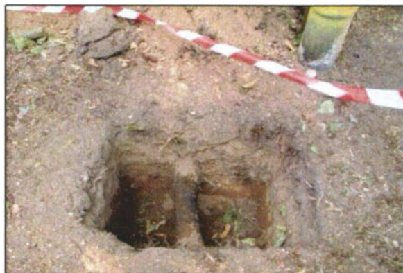
Photo 38: Where piles are proposed close to trunks, it is essential to excavate 50-75cm deep to see if there are any significant roots in the way, with provision to move the pile location if roots are found (note the pile was finally installed to avoid this root).
