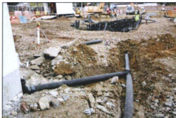
Photo 56: Drainage from adjacent buildings can be directed into Silva Cells, significantly buffering rainwater runoff from urbanised areas.
