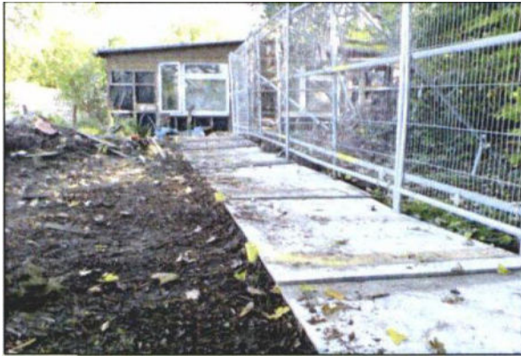
Photo 7: Heavy-duty plywood set onto a compressible woodchip layer and pinned into position is suitable to spread the loading from pedestrian access.
