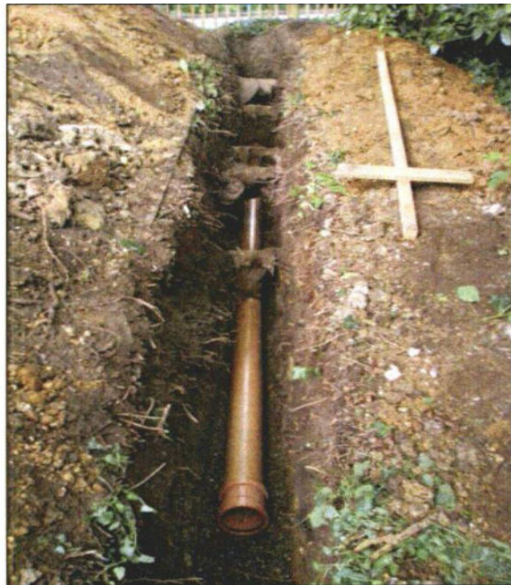
Photo 45: Continuous trenches dug by hand so that important roots can be retained (with the service ducting threaded beneath) is an effective means of minimising damage (note the ground protection boards with soil piled on top on the left).
