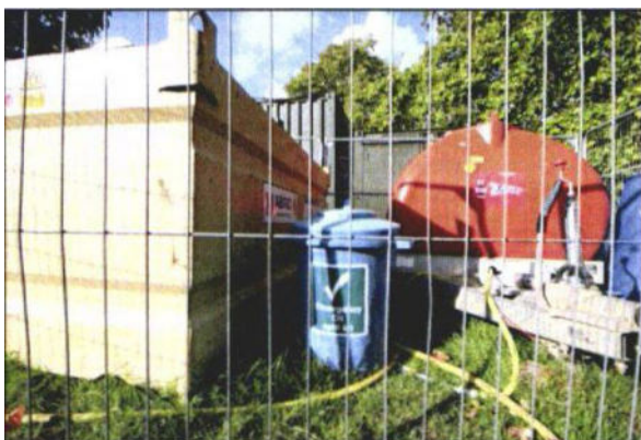
Photo 46: Where fuel or other chemical are stored on site, it is now standard practice to have emergency spillage kits available to restrict the environmental impact of accidents.
