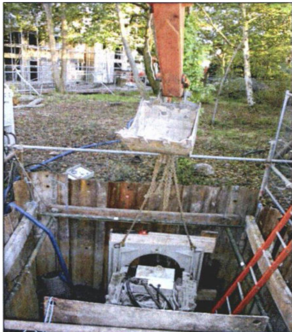
Photo 44: If possible, thrust boring is the preferred option for installing service routes through the RPAs of important trees, but there has to be space at the start and finish to dig substantial working pits.
