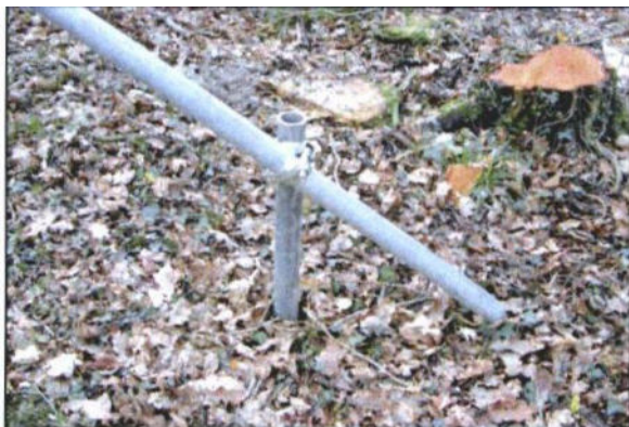
Photo 3: Close up of bracing detail, essential for increasing the stability of the vertical framework.
