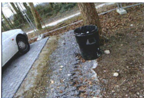
Photo 26: A conventional concrete haunching can be used to retain new surfacing as long as it is not dug into a trench – here is it placed on top of the CellWeb layer.
