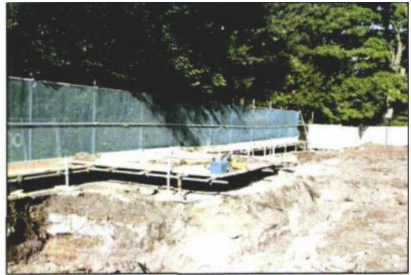
Photo 10: A scaffold framework attached to the main scaffold fencing can be used to support either scaffold planks or plywood to create an elevated platform with a gap beneath.
