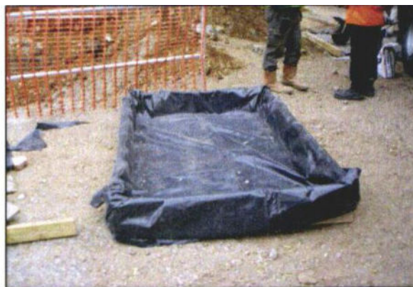
Photo 47: Soil bunding or a supporting framework covered in heavy-duty plastic sheeting is essential where there is a risk of spillages contaminating RPAs. This specifically applies to cement mixing areas and vehicle washing facilities.
