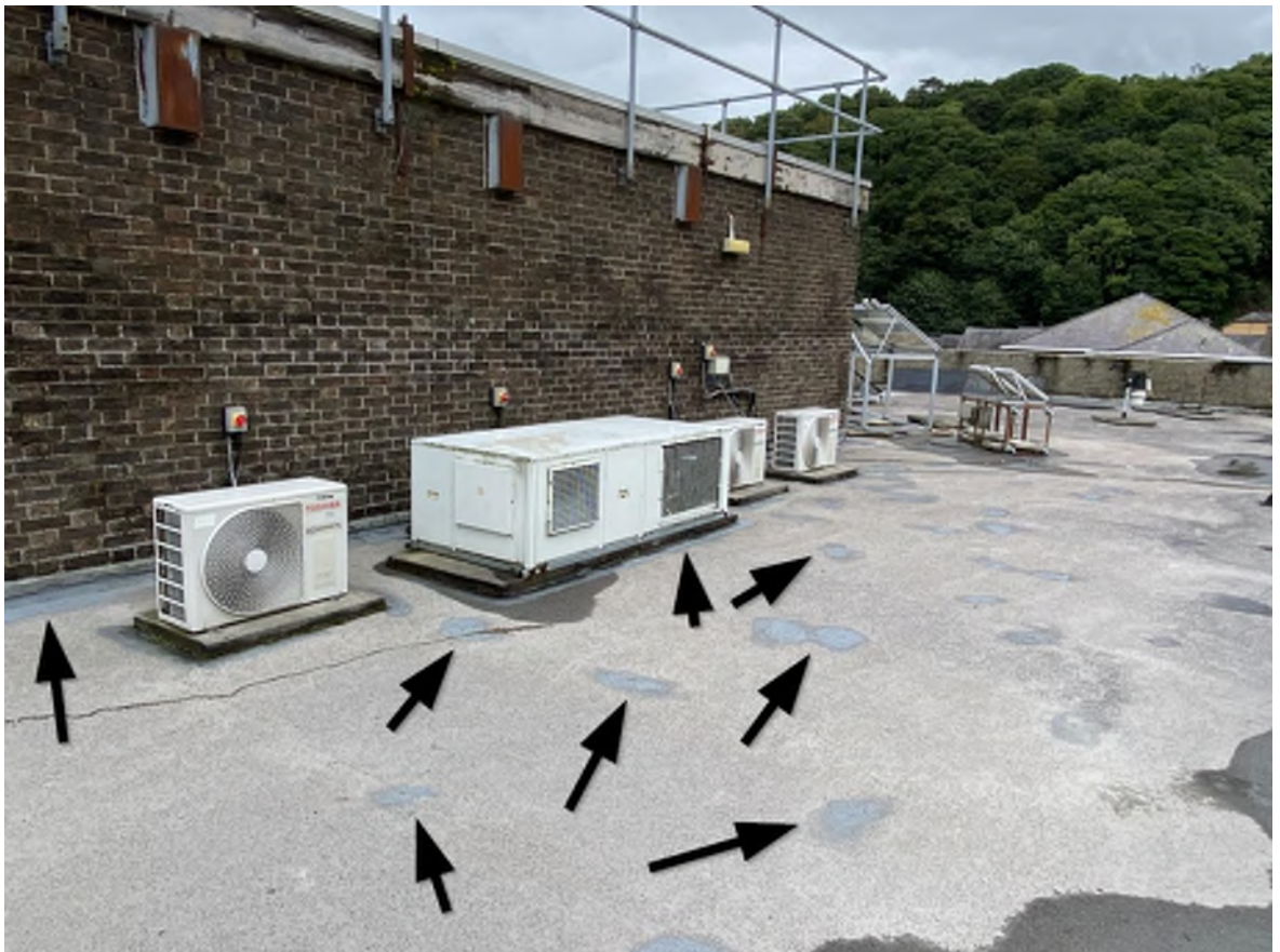
Photo of the engineering block roof showing patch repairs to felt roof covering.
