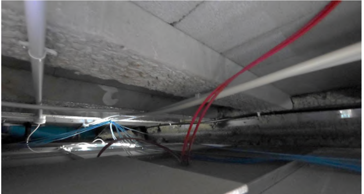
Photo of the existing Llwyn Brain ground floor ceiling void showing the underside of the beam & block floor construction and limited service distribution zone.
