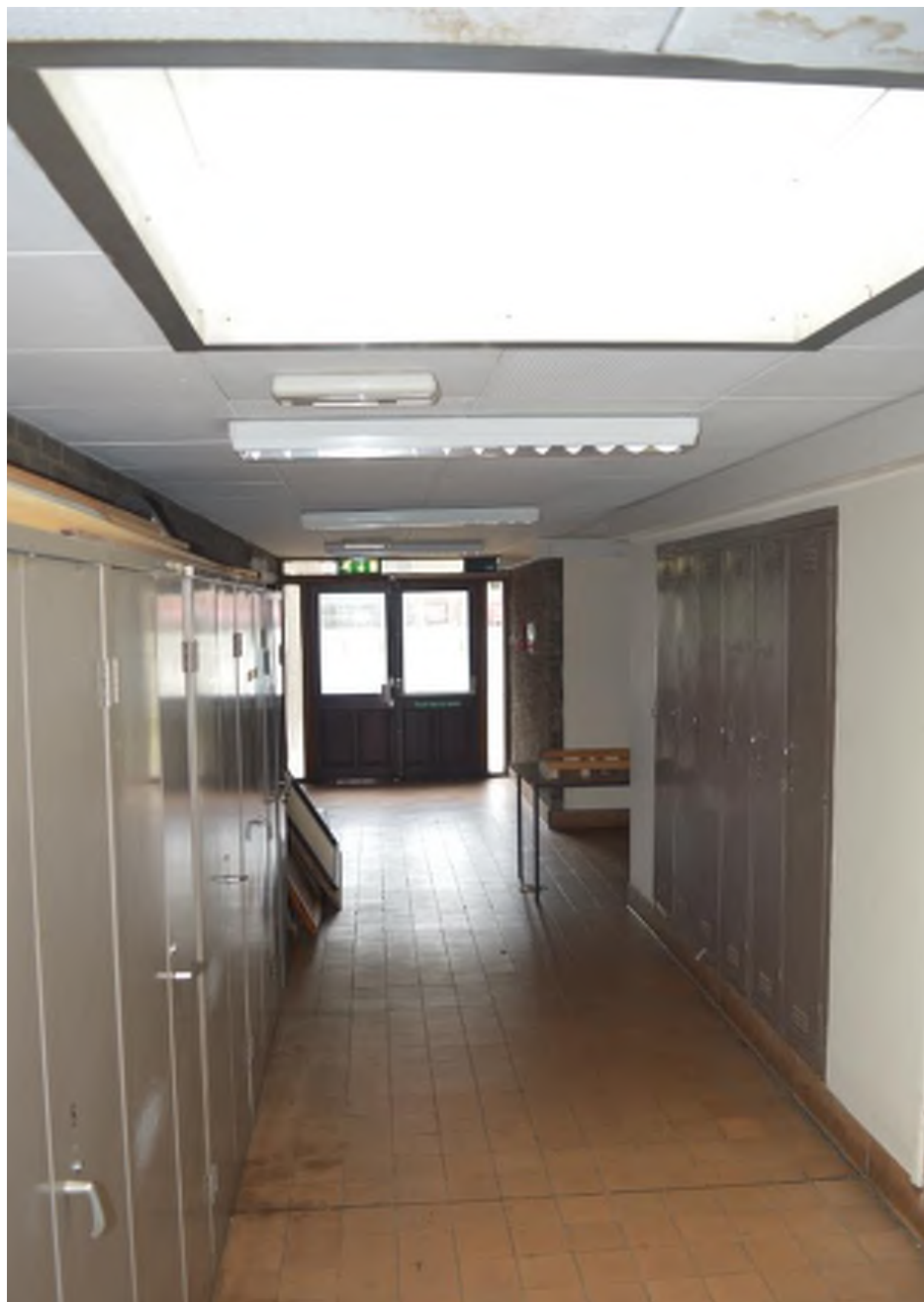
Photo of upper ground corridor to rear of engineering block showing rooflights to corridor and built-in lockers on plinths.
