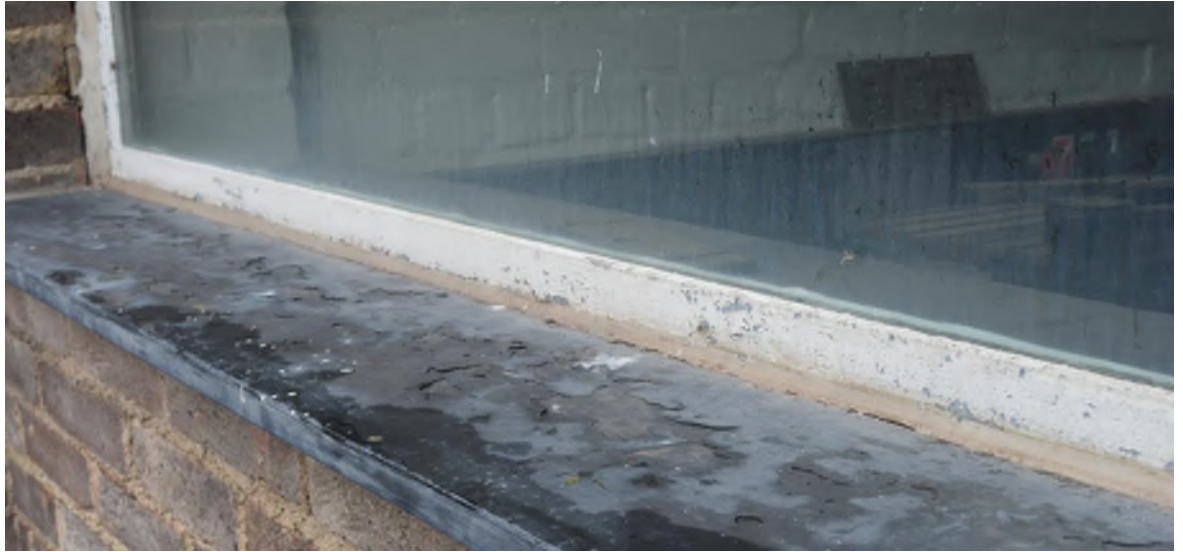
Photo of the single glazed uninsulated Crittal-type metal framed window system from outside.
