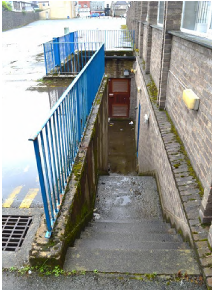
Photo of the lower ground (basement) SPEN HV substation access steps & louvred door.
